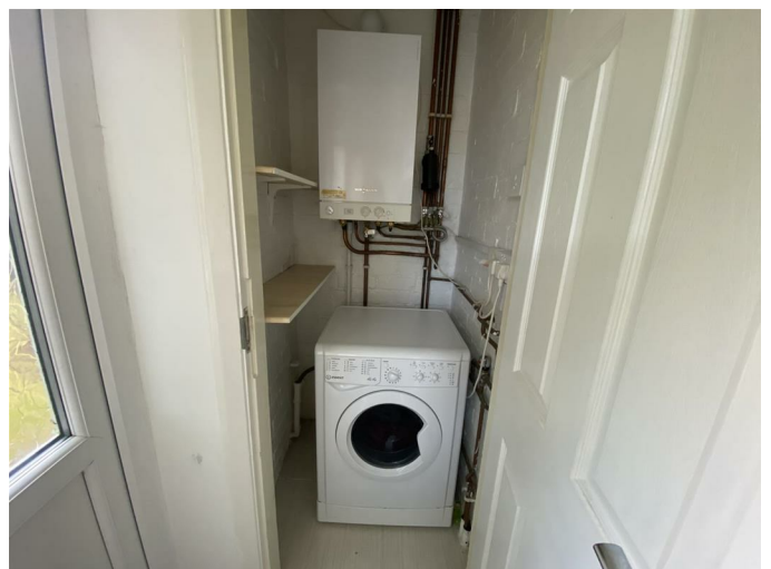
Utility Cupboard 4'2 x 3'3 (1.27m x 0.99m)
